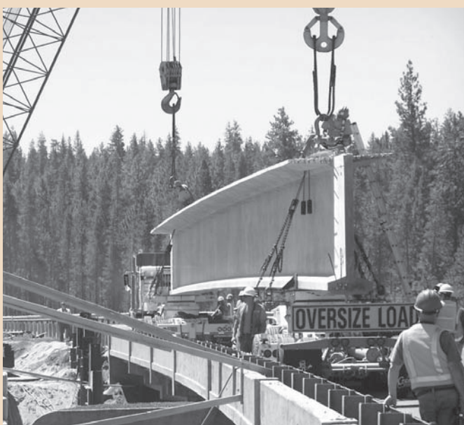
Bridge program contractors install one of seven record-breaking precast concrete beams—manufactured in-state—at the Union Pacific Railroad overcrossing near Chemult, Oregon.
