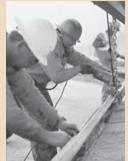
Workers install a guardrail along US-97 during the first stage of the Oregon bridge program.
